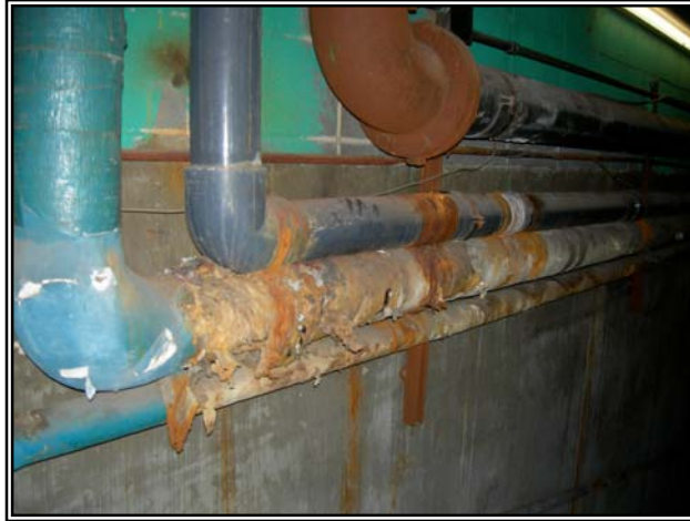
Building systems in disrepair are a common sight at Ridgeland Common and cause many day to day maintenance issues. Unfortunately, undertaking extensive renovation/repair is costly and time consuming.
